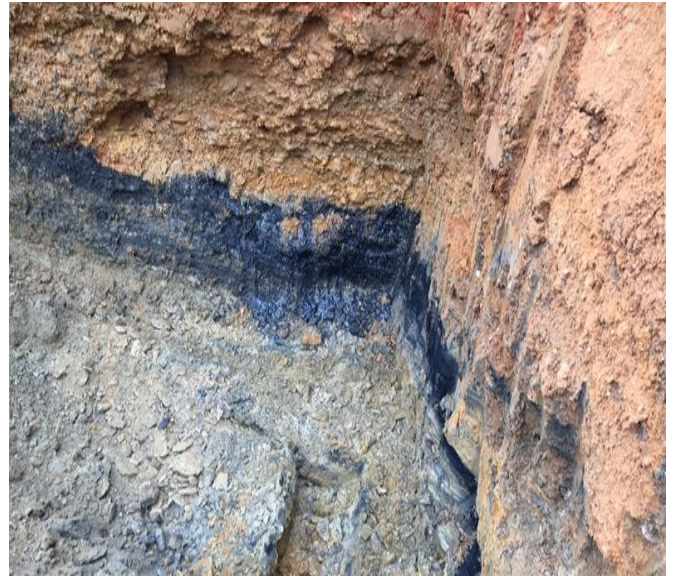
Impacted soil seam and LNAPL in excavation of elevator shaft
