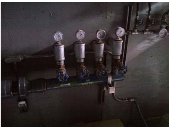
REMEDIATION SYSTEM – VAPOR EXTRACTION MANIFOLD
