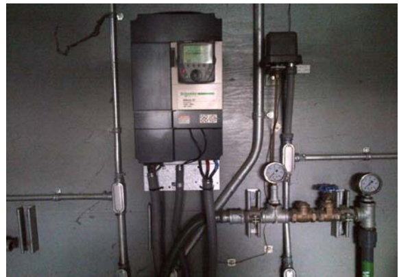
REMEDIATION SYSTEM – CONTROL UNIT
