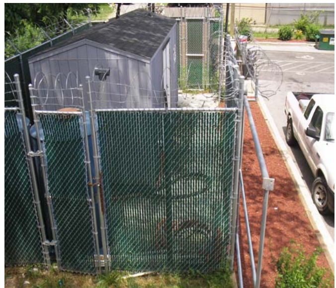
REMEDIATION SYSTEM ENCLOSURE AT SITE
