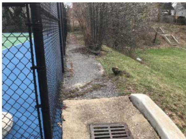
Tennis court inlet
