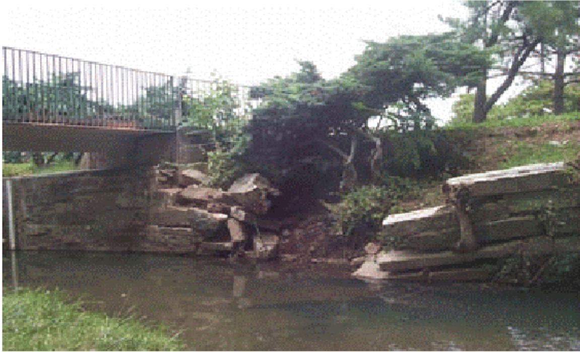
Picture taken from the District's TMDL Report. High flows probably scoured under the wall's footing causing the collapse.
