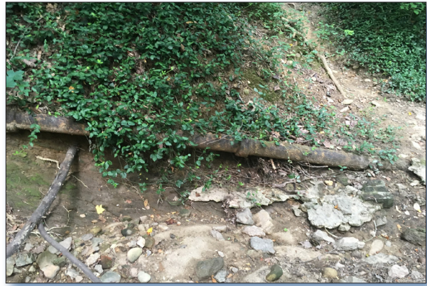
Figure 3. Sewer pipe exposed by erosion.
