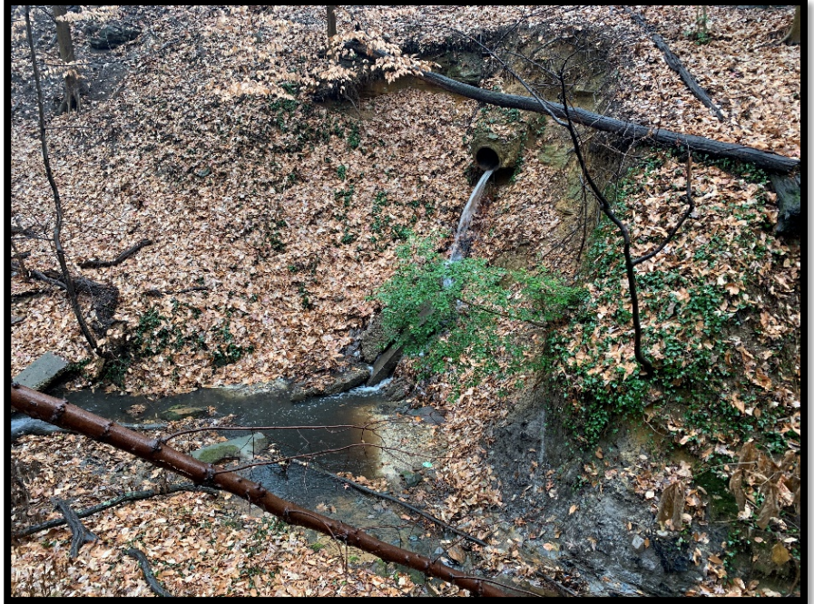
Figure 4 - Eroded outfall at Park Drive to be repaired in FY 2023.
