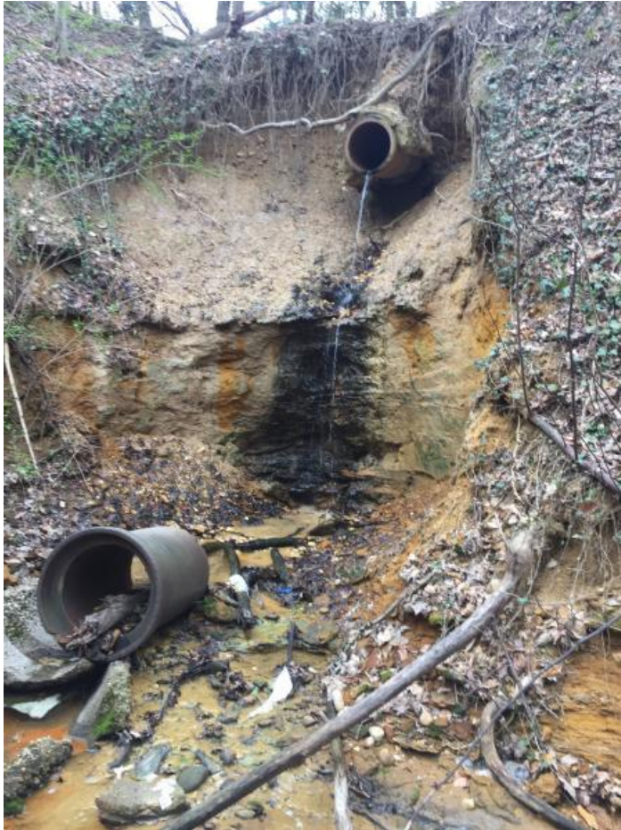
Figure 5 – Outfall to be repaired as part of Park Drive Gully Restoration
